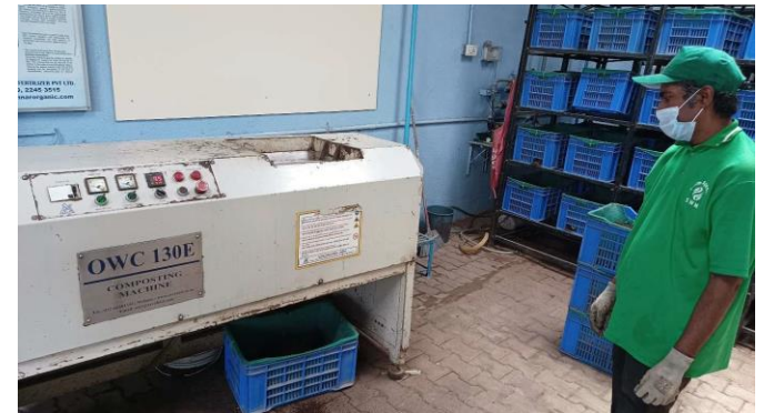
The Organic Waste Converter (OWC) facility on the campus of Global Infocity park, Chennai
